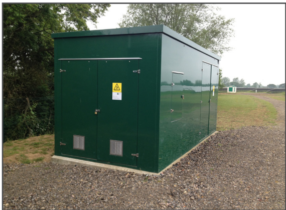
Plate 6.6 - Typical GRP Cabinet
