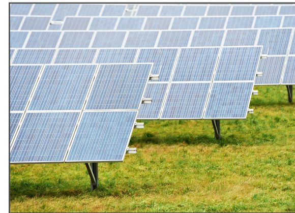
Plate 6.1 - Typical Ground-Mounted Solar Array on Frame with Anchors
